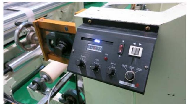
Remote Controller is installed on Slitting Machine by Wall-Mounted
